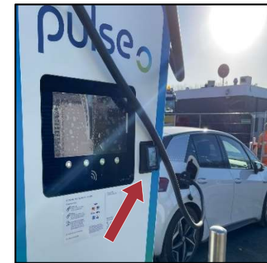
Electric Vehicle Charging Station
